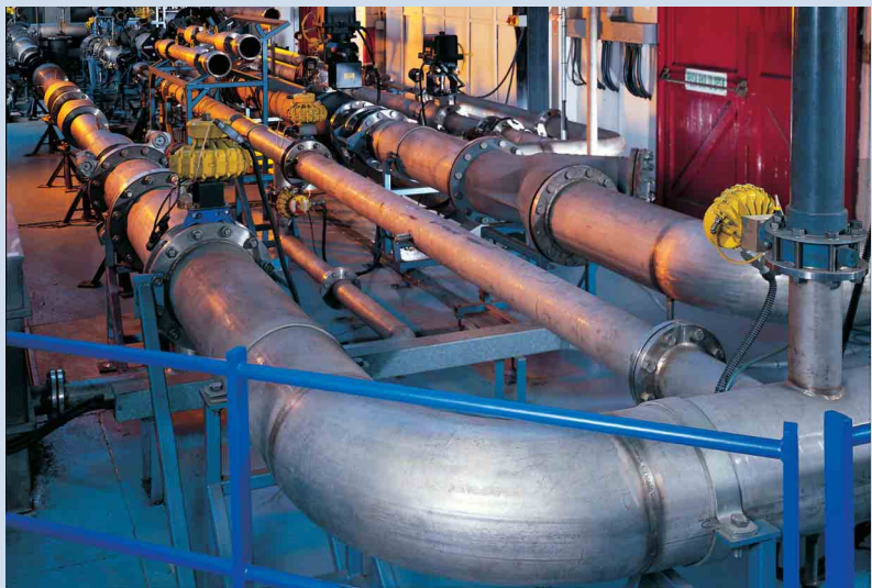
Flowmeter calibration rig, Spirax Sarco, Cheltenham, UK.
